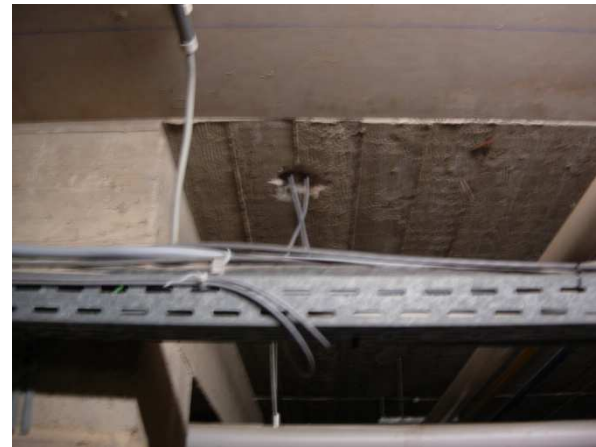
> 60m cables in data cables pathways
